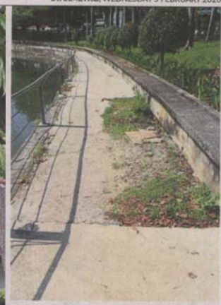
Regulars to Taman Jaya say the broken jogging path is a safety hazard. — Filepic
