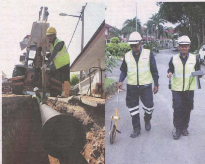
A total of RM161.9 million was spent in 2019 for replacement works of 168.34 km of old and frequently burst pipes. Photo on the right- Leak detection works.
